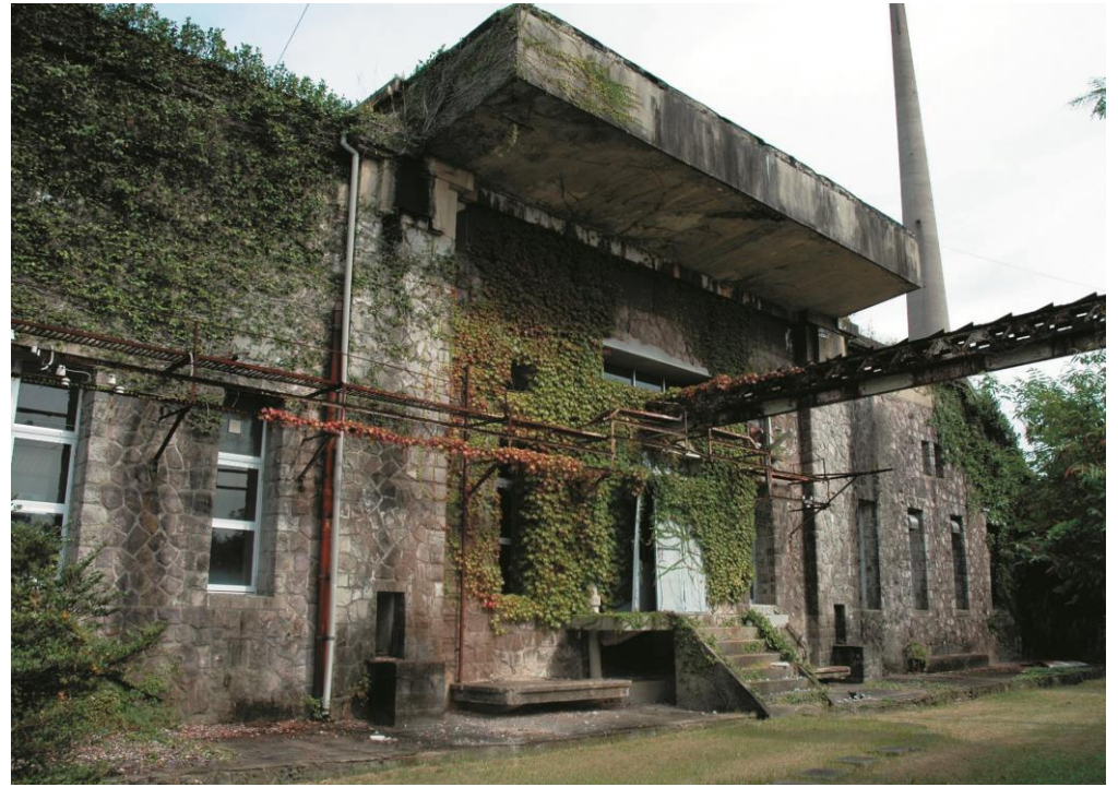
Fig.5 The current transmission room
